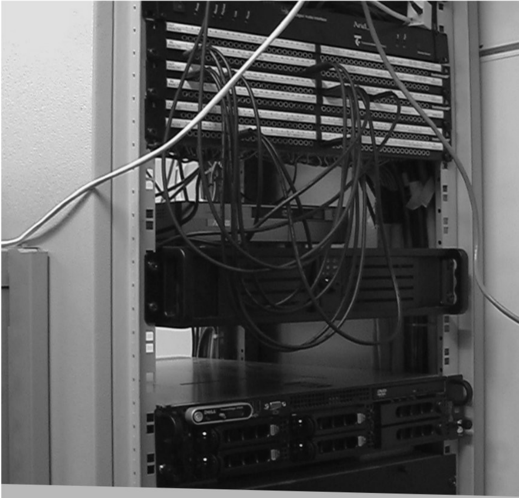
An analog studio – devices are connected with cables.
